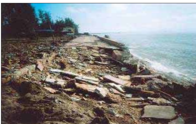
Fig. 10. Concrete sea dykes in Do Son Town (Hai Phong Prov.) were broken by heavy storms
